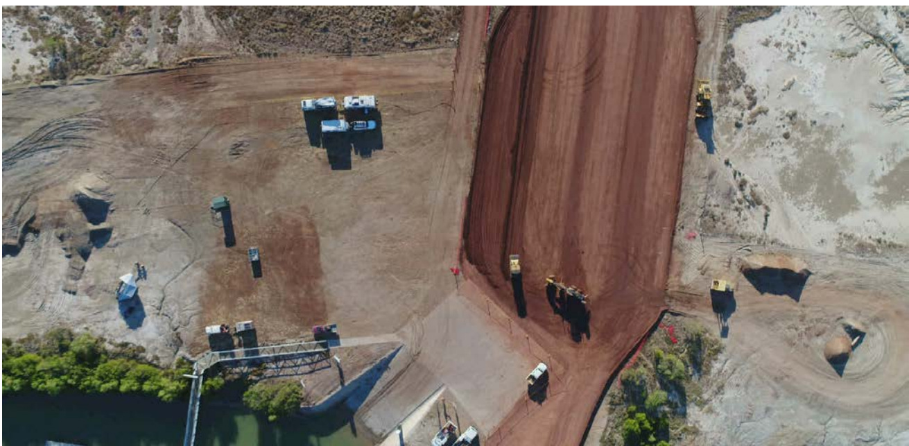
Image: Burketown Wharf Boat Ramp and Car Park Construction. This project was completed in July 2018.
